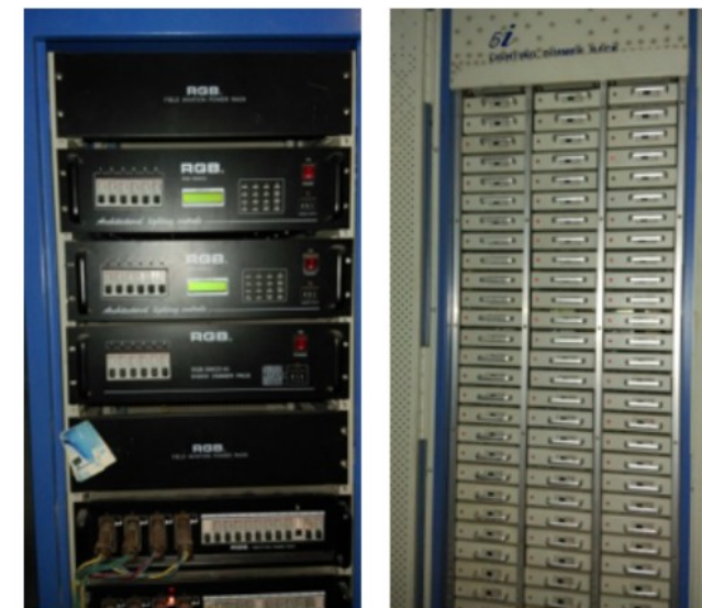
Lighting control cabinet
